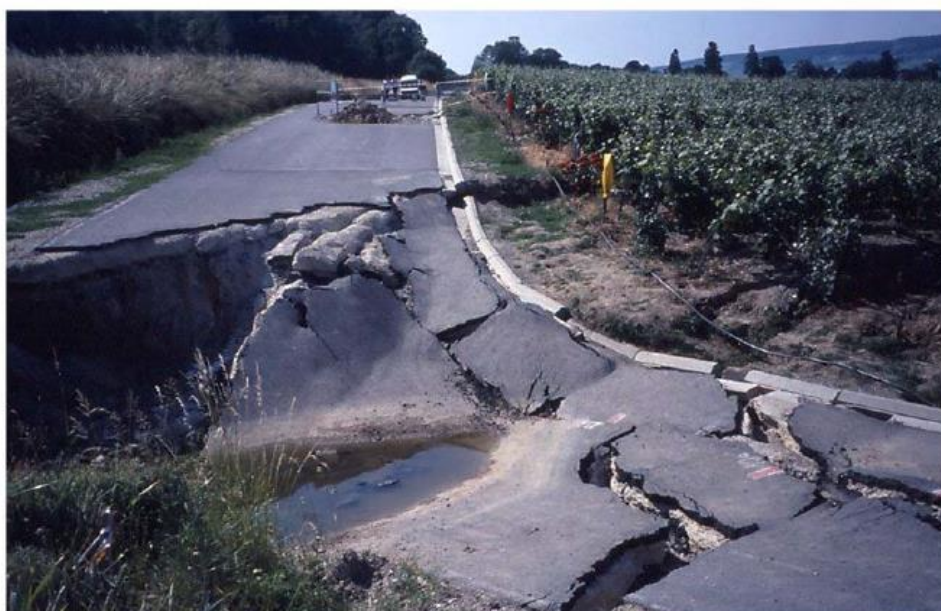
Figure 4 – Landslide affecting Champagne “terroir”, near Reims (France).
